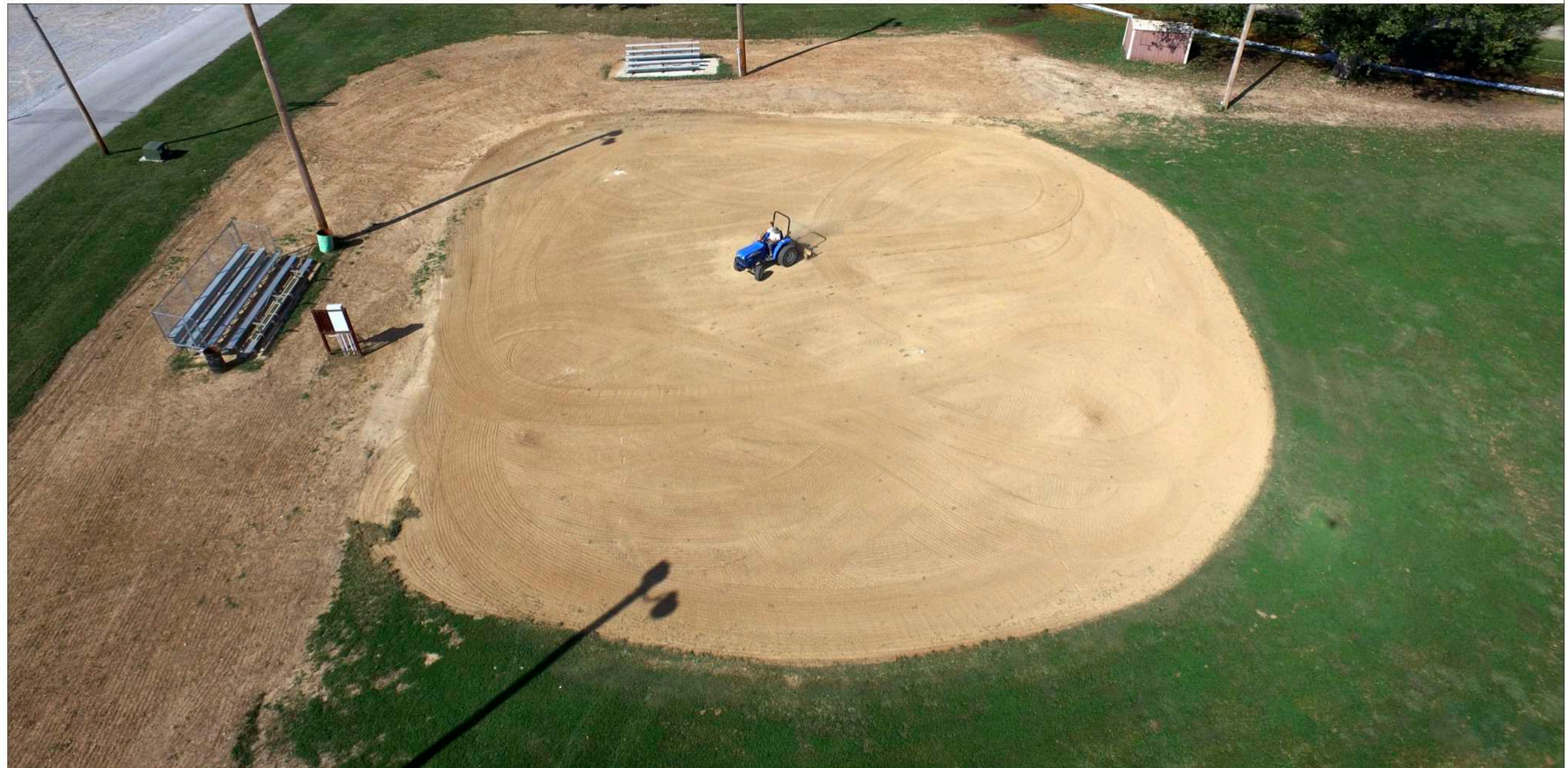
RIGHT • In this drone photo, Bernie Kim, a Perryville Parks employee, removes grass from an under-construction baseball field.
